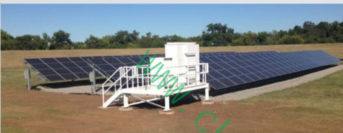
Figure 25: 86kW PV Array
