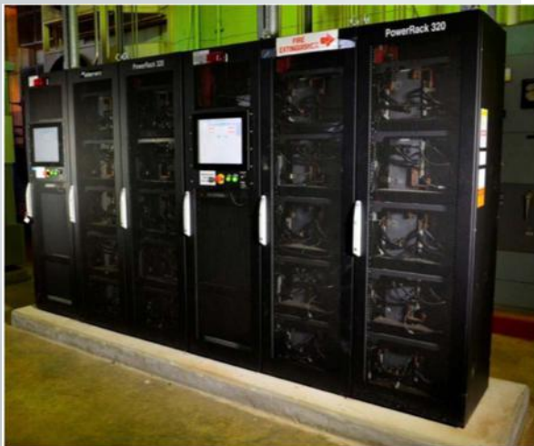
Figure 27: 400kW Power Optimized Storage Battery
